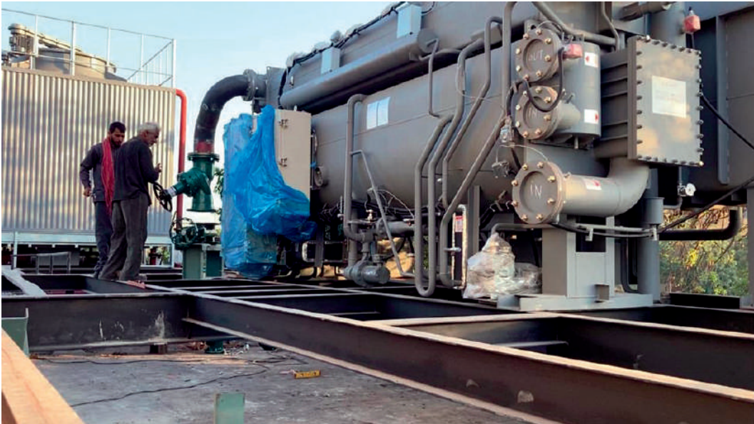
The cogeneration system in SB #01 & SBASSE using a gas generator fuel system
